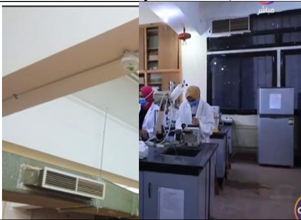
6. Example of presence of chimneys with filters for research devices (Faculty of Pharmacy, Beni-Suef University, Beni-Suef)
