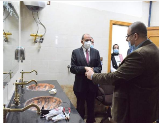
7. Using water taps that operate with sensors (Beni-Suef University , Beni-Suef)
